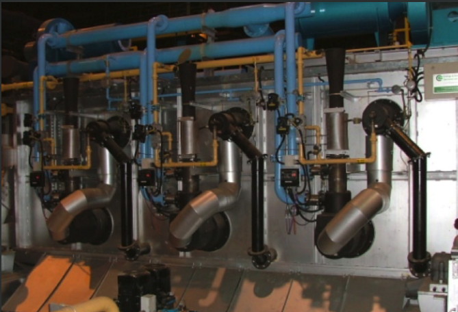
Fig. 3 Furnace burners & recuperators.
