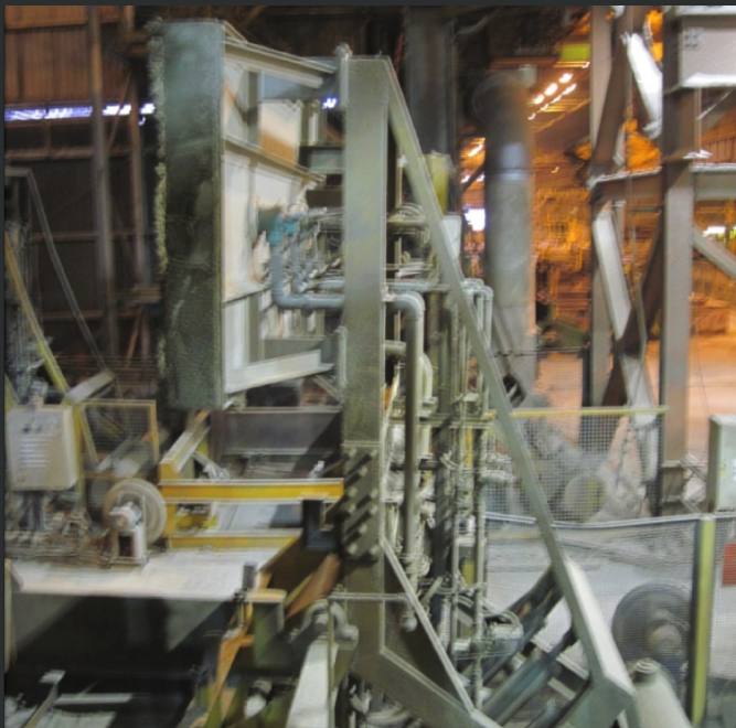
Fig. 3 Modified Combi-Caster Dryer with 3 Burners.
