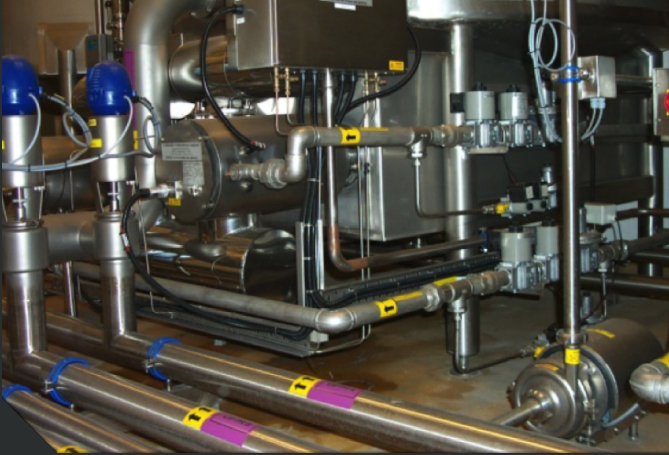
Fig. 1 Gas supply, controls and pipework.
