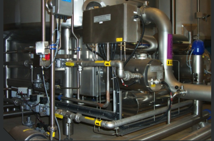
Fig. 2 Gas supply, controls and pipework.
