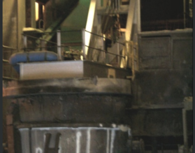
Fig. 2 Dual fuel burner and long view of heater with ladle in the working position.
