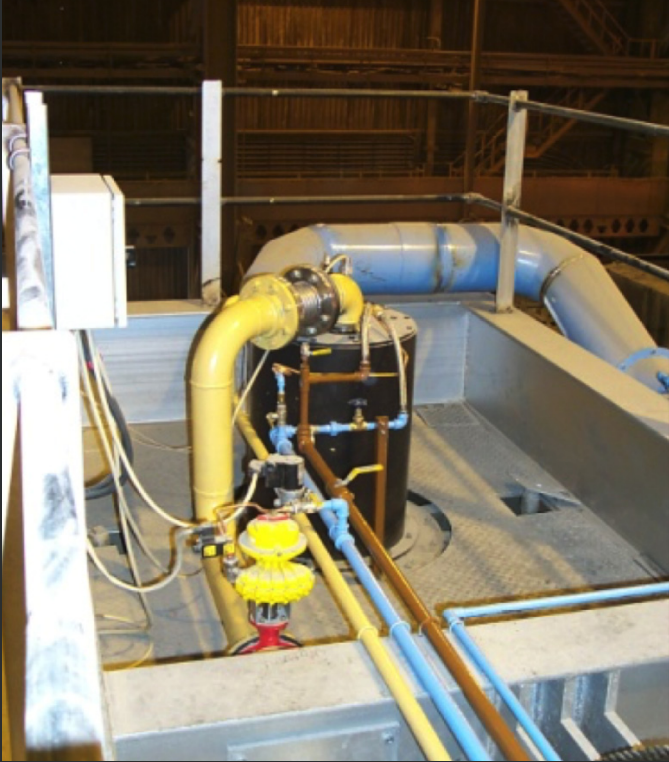
Fig. 1 Dual fuel burner and long view of heater with ladle in the working position.
